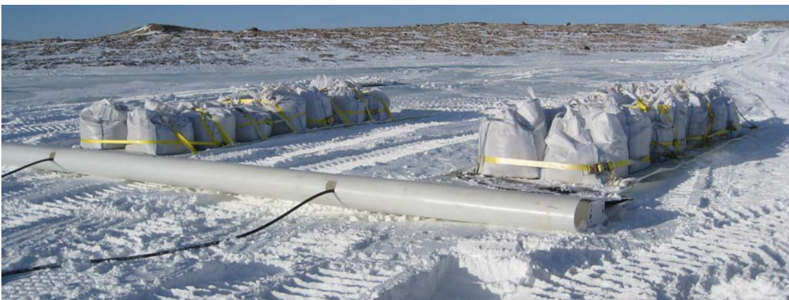
Figure 12. New spreader bar consisting of square-section steel tubing wrapped with a sheet of HMW-PE to form a curved nose and to support bladder- and cargo-sled tow plates.
