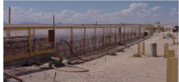
Figure 6. Helium bag over pulldown
