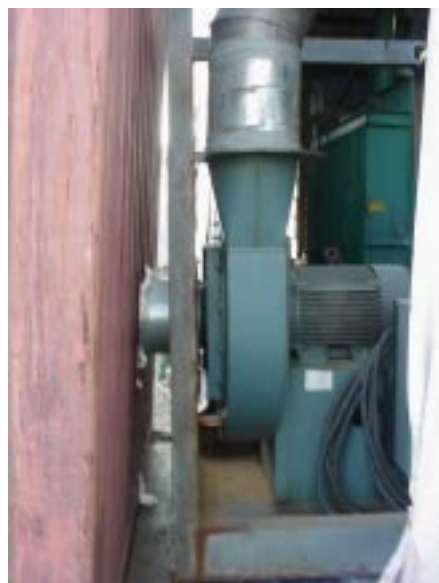
Figure 2: Test Chamber Ventilation Fan
