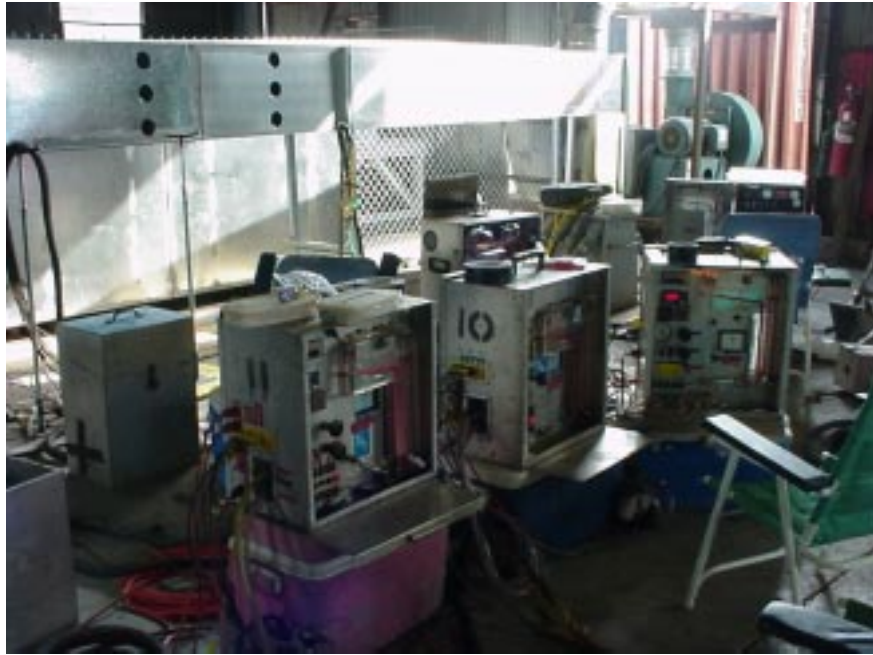
Figure 3: Sample Duct and Equipment
